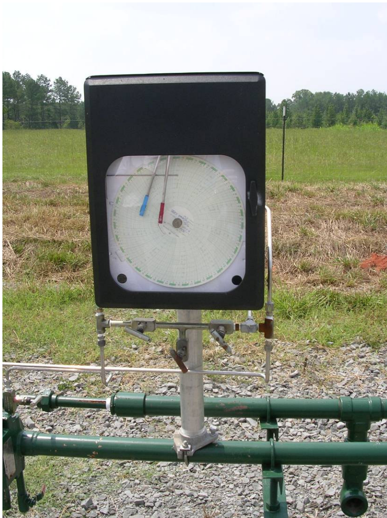
Figure 6-4. Flow Meter Used on CBM Wells.
