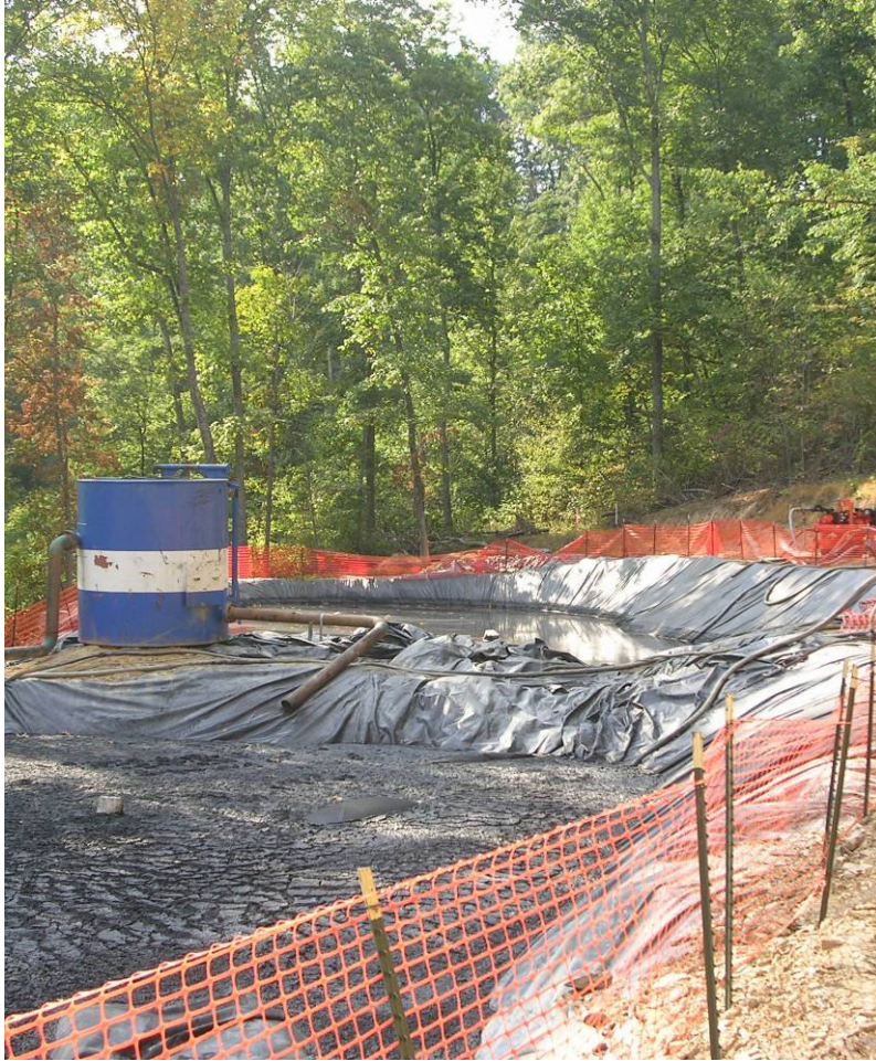
Figure 6-11. Mixing Tanks for Drilling Fluid Treatment
