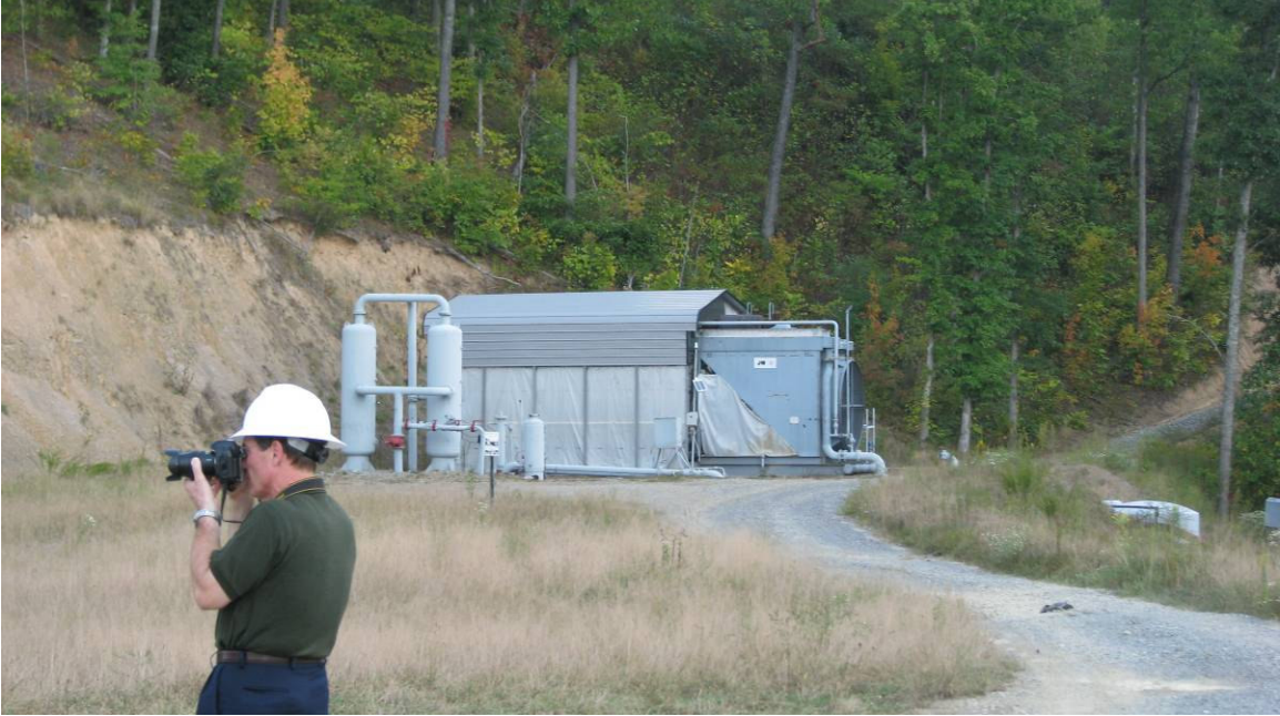
Figure 6-3. Pinnacle 97 Compressor Station.
