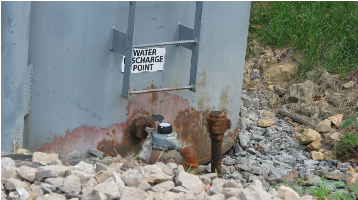
Figure 6-7. Wastewater Discharge Point
