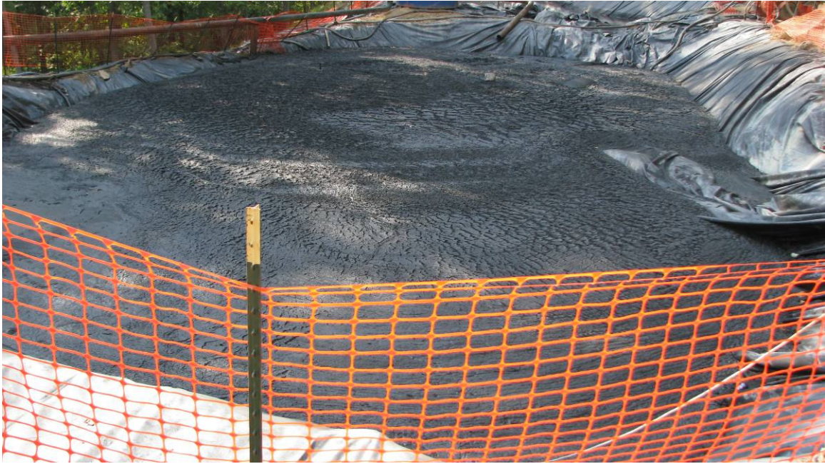
Figure 6-13. Secondary Settling Lagoon for Drilling Fluid
