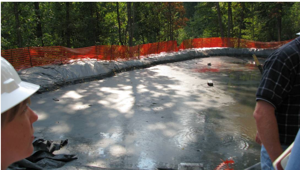
Figure 6-12. Primary Settling Lagoon for Drilling Fluid
