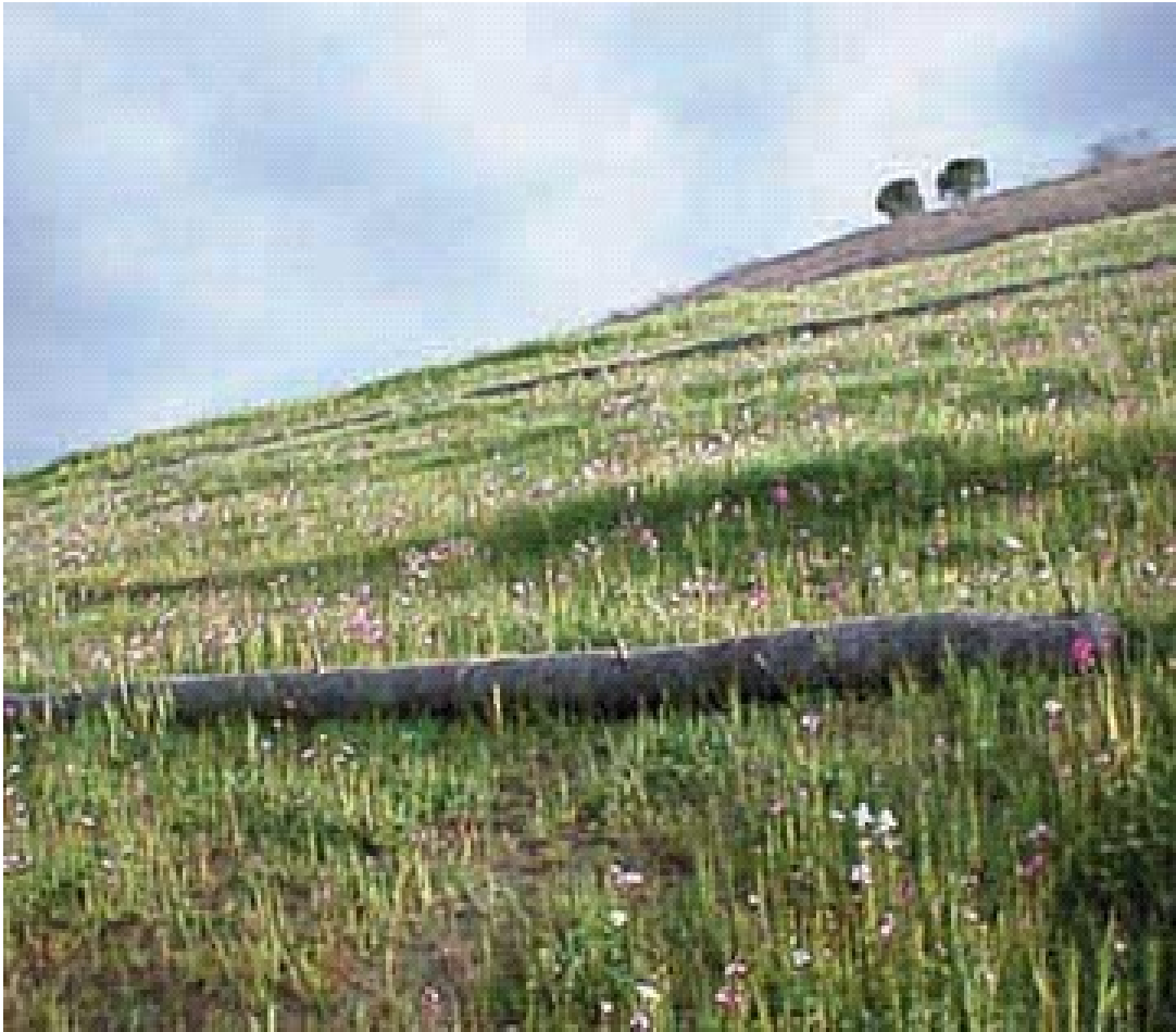
Fiber rolls along a newly-vegetated hillside. Note the disturbed slope at the top of the hill Source: EPA Storm Water Menu of BMPs, 2004
