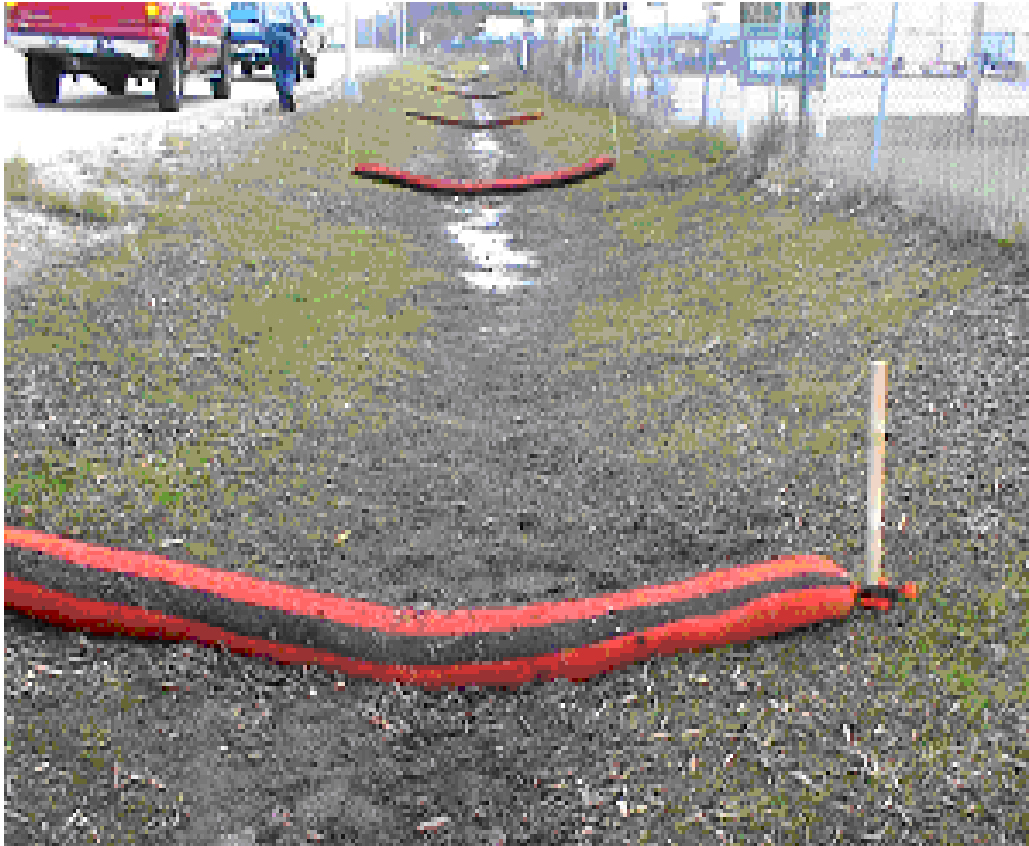
Compost Socks staked in place along a storm water swale. Source: Ohio Department of Transportation, 2008
