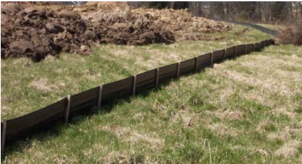
Properly installed silt fence along a disturbed slope. Note the use of vegetated buffer and the tight spacing of posts.
