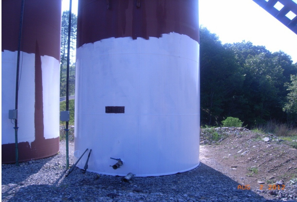
Figure 11: Flowback Sampling Point at Condensate Tanks, Donna Pad
